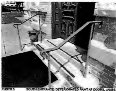
PHOTO 3 SOUTH ENTRANCE: DETERIORATED PAINT AT DOORS, JAMBS, AND HANDRAIL. BIOLOGICAL STAINING AT STEPS
