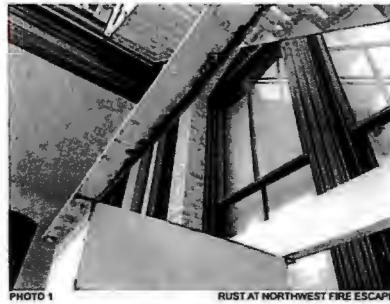
PHOTO 1 RUST AT NORTHWEST FIRE ESCAPE
