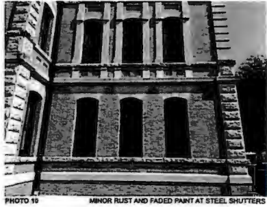
PHOTO 10 MINOR RUST AND FADED PAINT AT STEEL SHUTTERS
