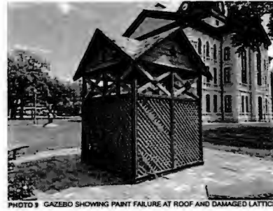
PHOTO 9 GAZEBO SHOWING PAINT FAILURE AT ROOF AND DAMAGED LATTICE
