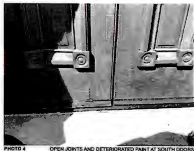
PHOTO 4 OPEN JOINTS AND DETERIORATED PAINT AT SOUTH DOORS
