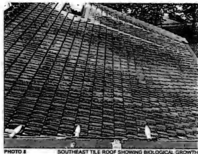
PHOTO 8 SOUTHEAST TILE ROOF SHOWING BIOLOGICAL GROWTH
