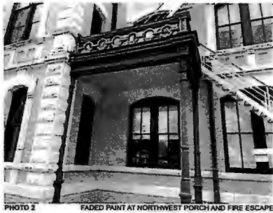
PHOTO 2 FADED PAINT AT NORTHWEST PORCH AND FIRE ESCAPE
