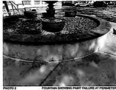
PHOTO 5 FOUNTAIN SHOWING PAINT FAILURE AT PERIMETER
