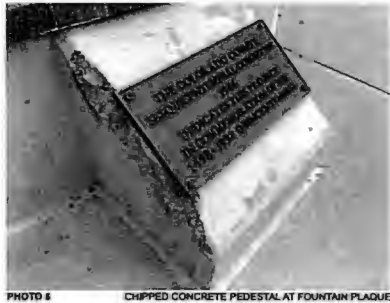
PHOTO 6 CHIPPED CONCRETE PEDESTAL AT FOUNTAIN PLAQUE
