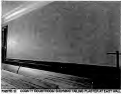
PHOTO 11 COUNTY COURTHOUSE SHOWING FALLING PLASTER AT EAST WALL
